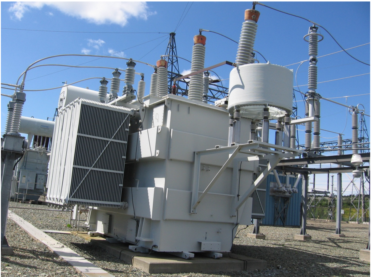
Figure 1: Power Transformer T4 at Hardwoods Terminal Station
