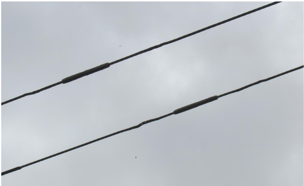
Figure 7 – #2/0 ACSR Conductor with Compression Sleeves and Bird Caging
