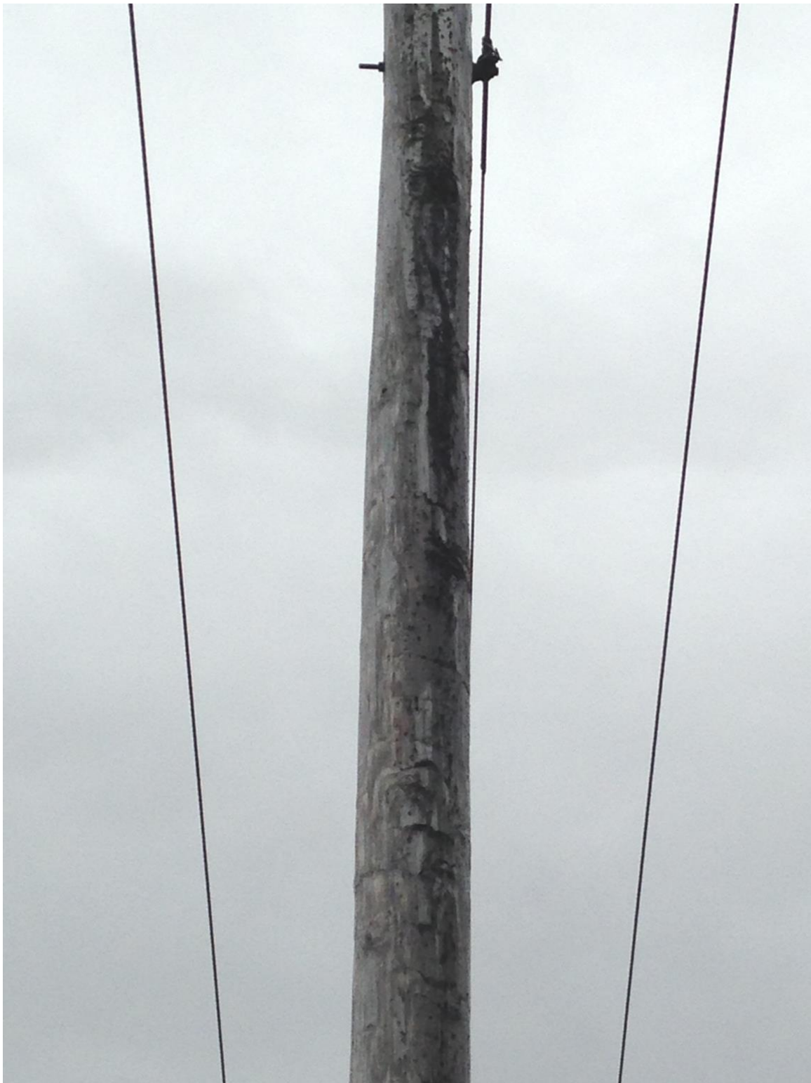
Figure 3 – Burn Damage on Pole due to Insulator Failure
