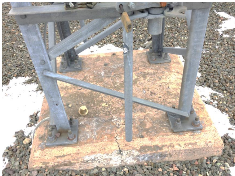
Figure 8: A Pier Foundation that Requires Refurbishment
