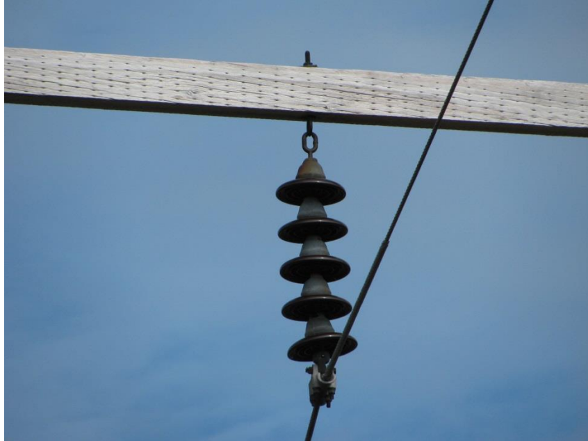
Figure 8 – Original Vintage COB Porcelain Insulators
