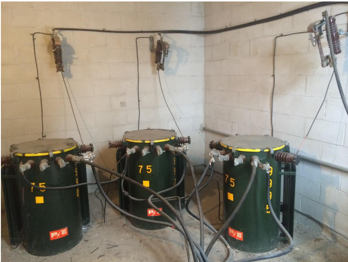
Figure 2: Forest Hill Apartments Pole Mount Transformers
