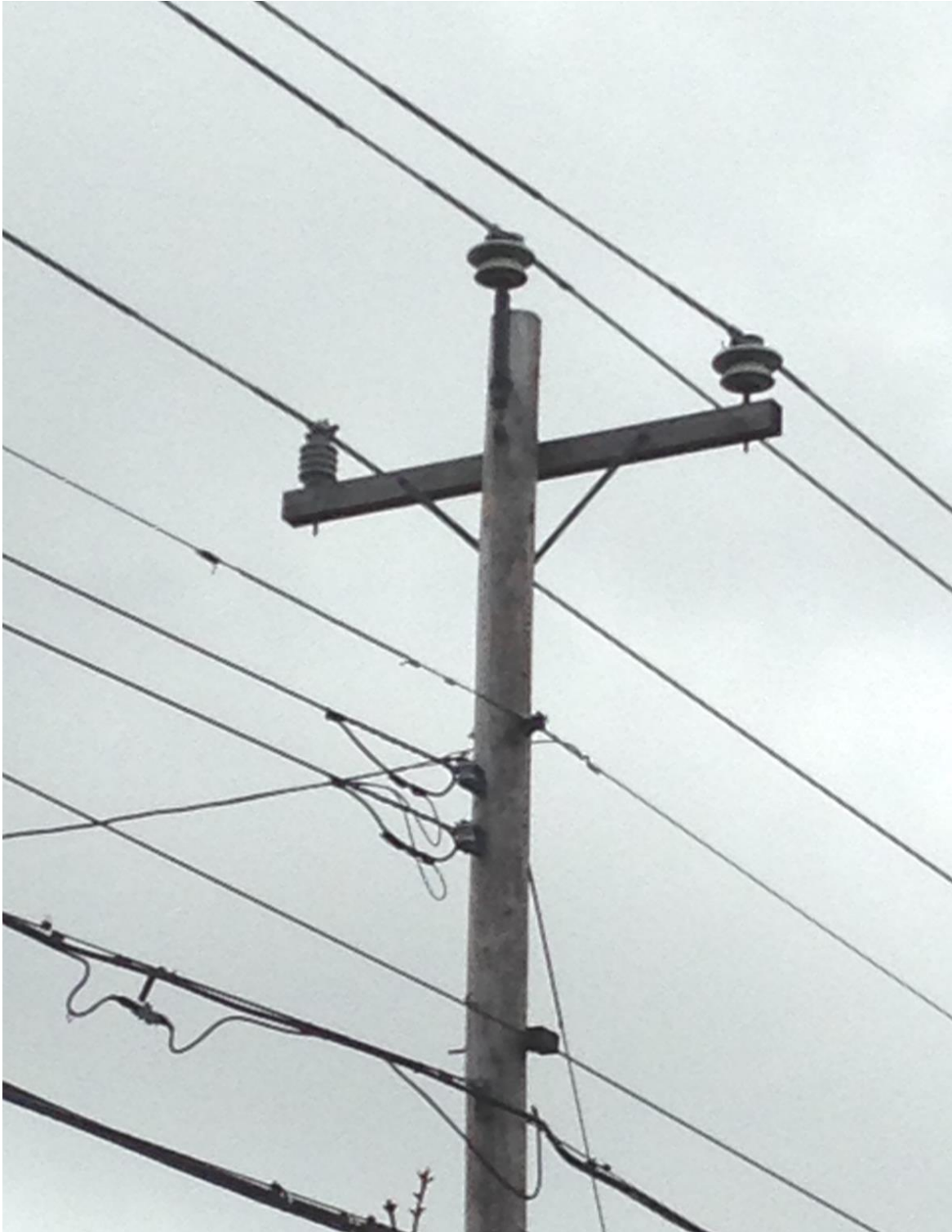
Figure 1 – 2 Piece Insulators with 1 Previous Failure
