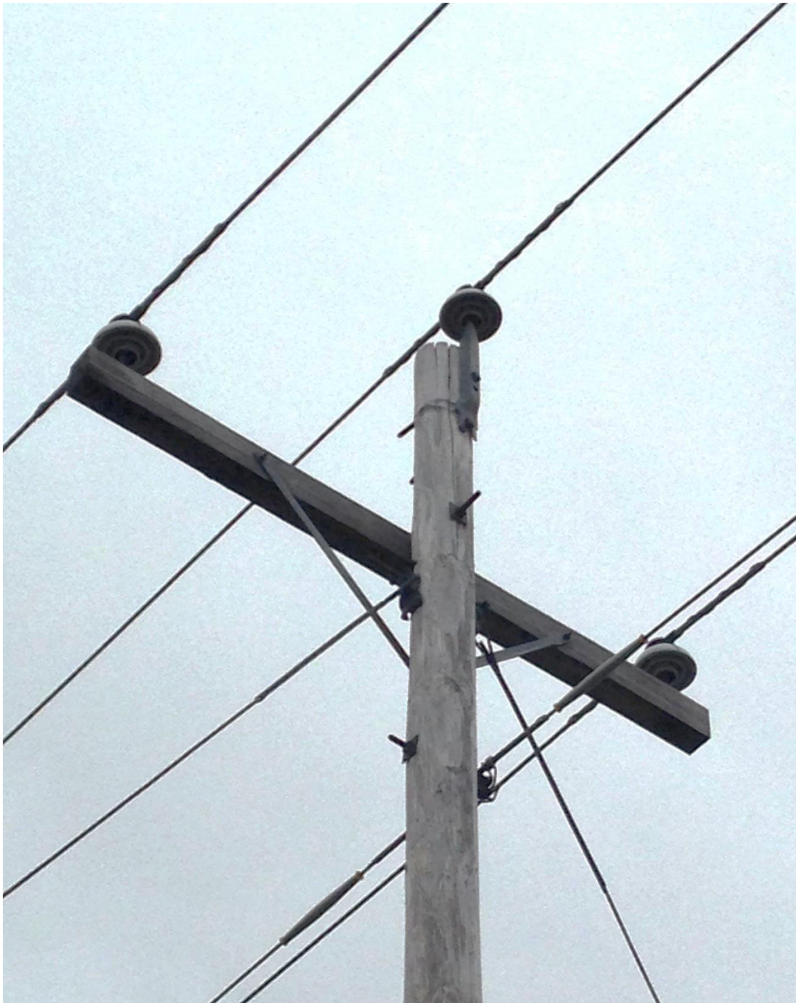
Figure 5 – Pole Top Deterioration
