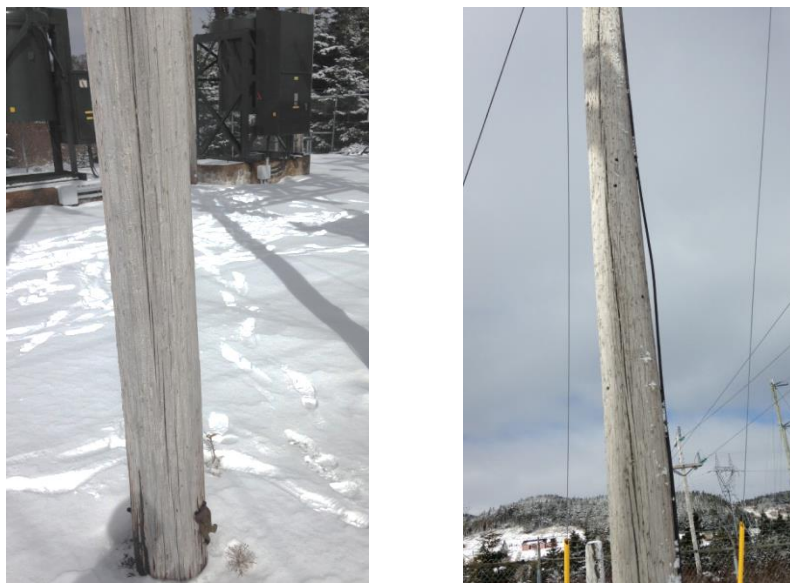
Figure 2: Deteriorated Wood Poles
