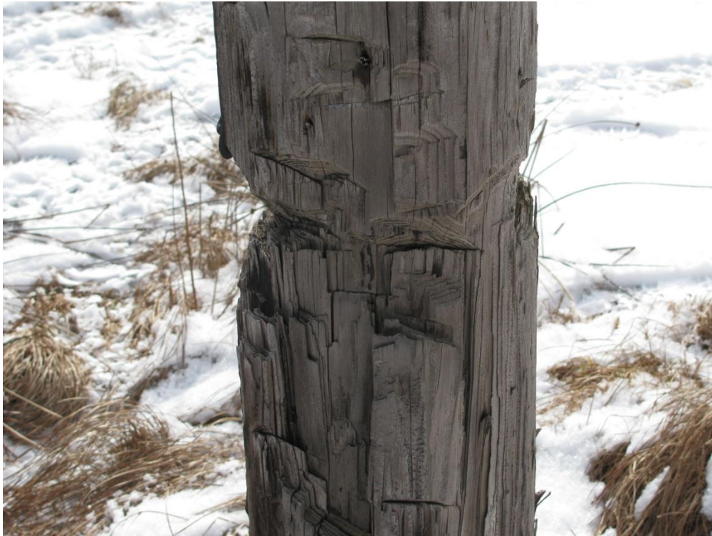
Figure 14 – Vandalism - Pole Damage
