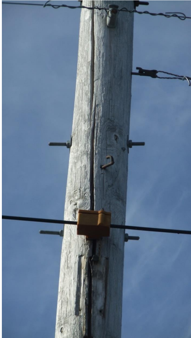
Figure 5 – Bolts Provide Temporary Repairs to Damaged Pole
