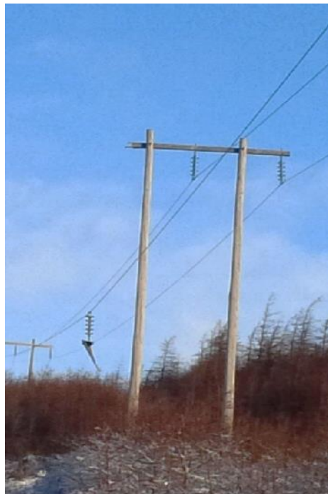
Figure 13 – Damage Resulting from Rotten Crossarm
