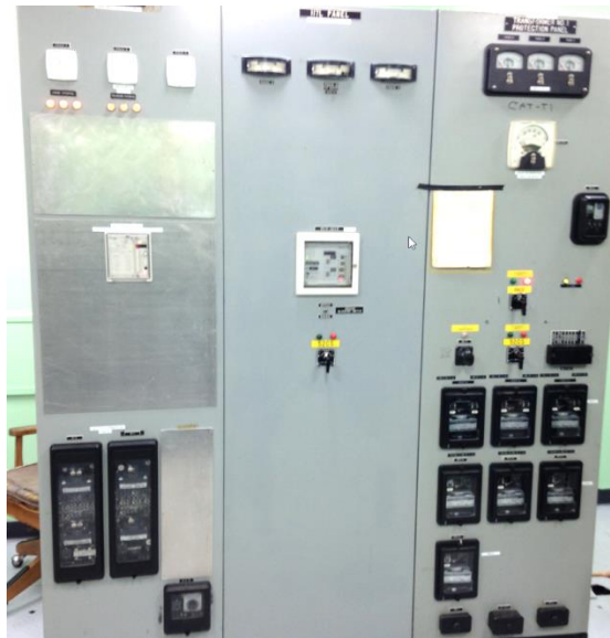
Figure 11: Existing Control Building with Electromechanical Relays
