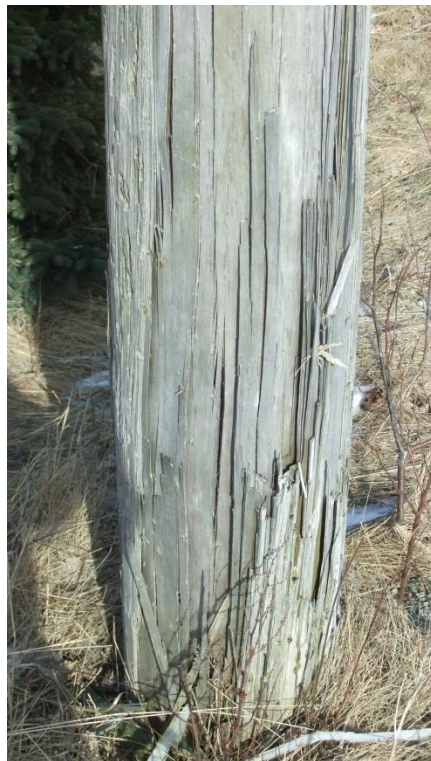
Figure 2 – Pole Shell Layer Separation
