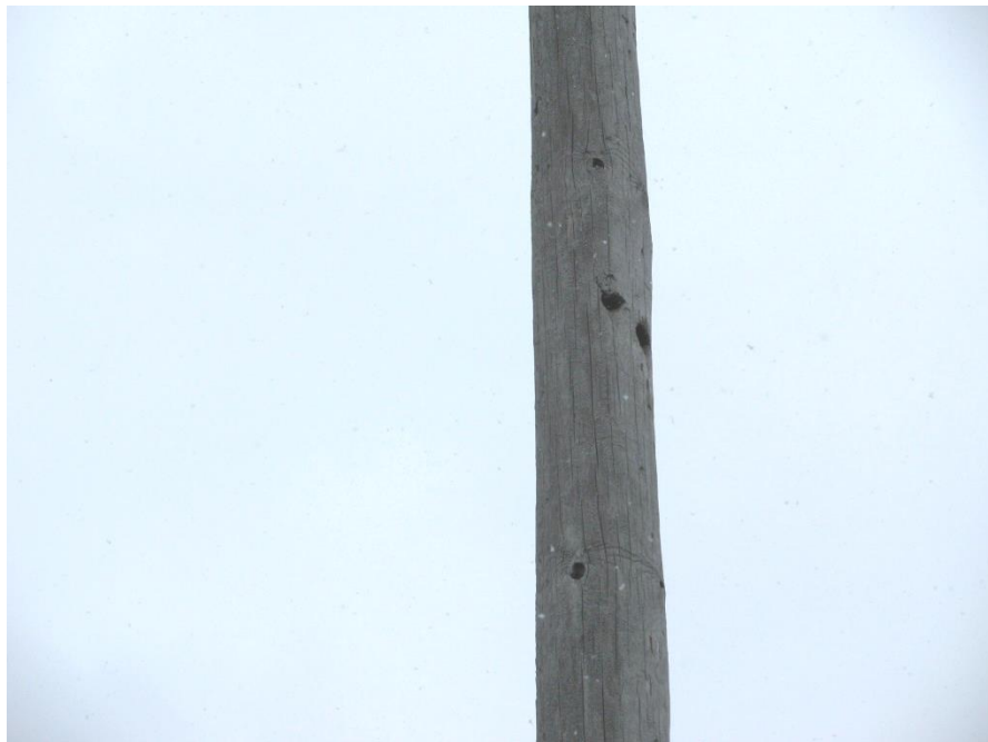
Figure 15 – Woodpecker Hole Damage
