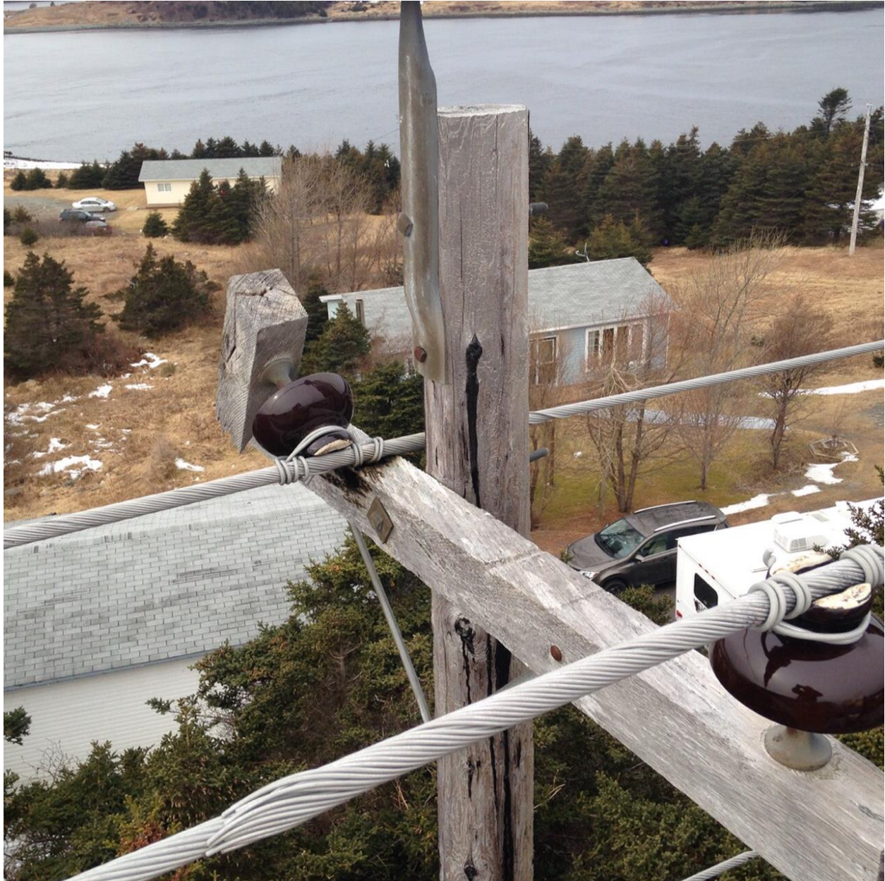
Figure 7 – Outage Cause by Deteriorated Crossarm
