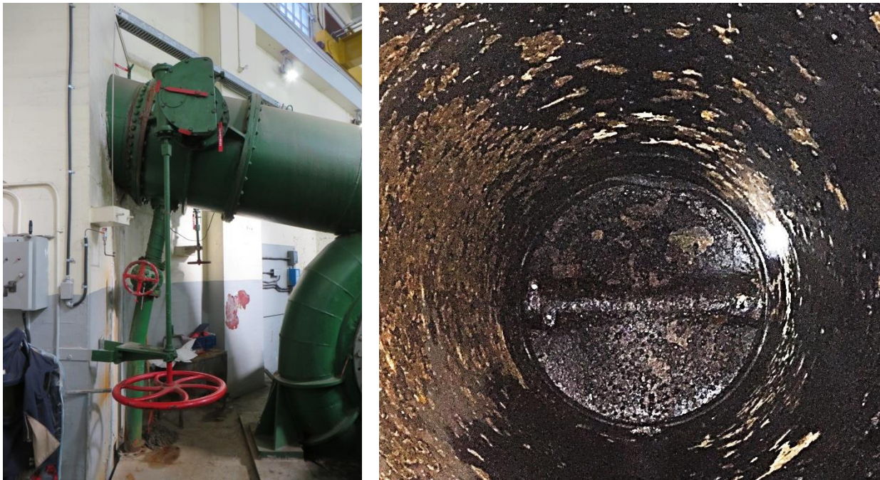
Figure 3 – G1 Valve Exterior Setup and G3 Valve Seal Separation
