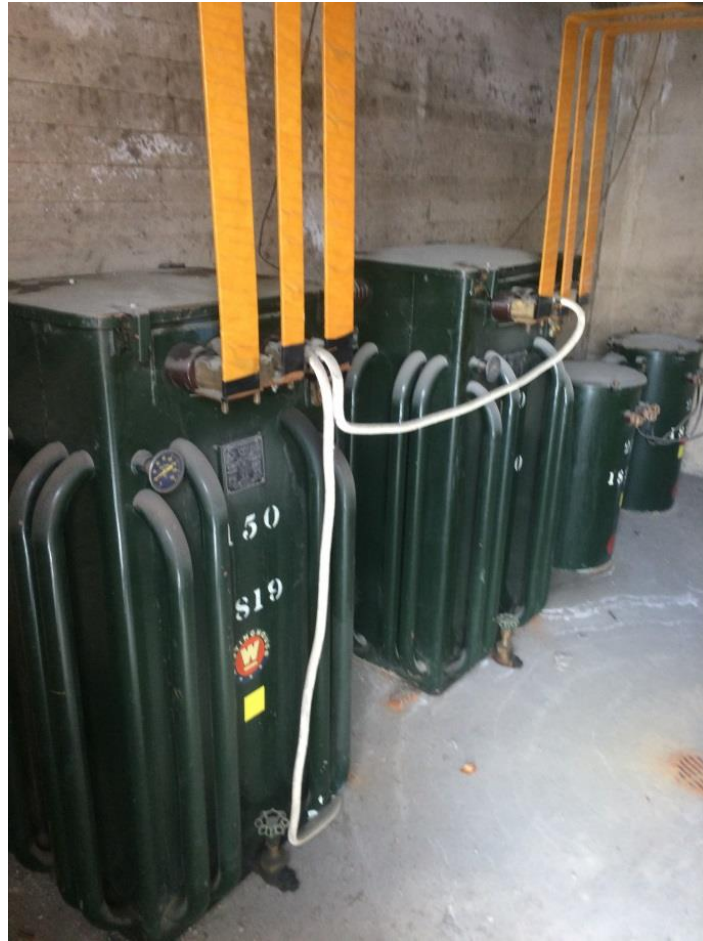
Figure 7: Churchill Square Apartments Pole Mount Transformers
