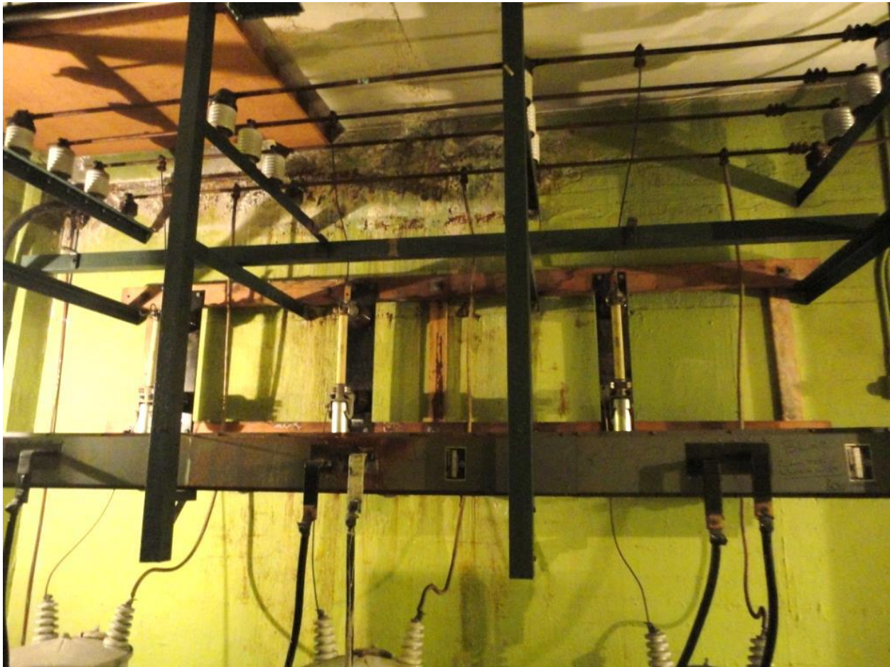
Figure 5: TNT Building Pole Mount Cutouts
