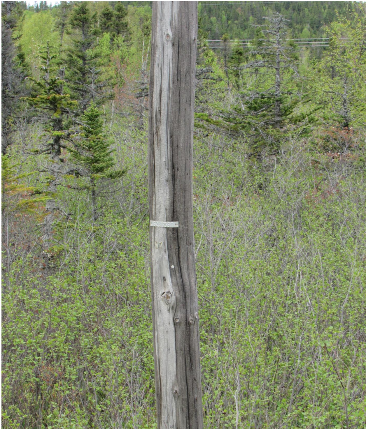
Figure 2 – Bent Pole with Checks
