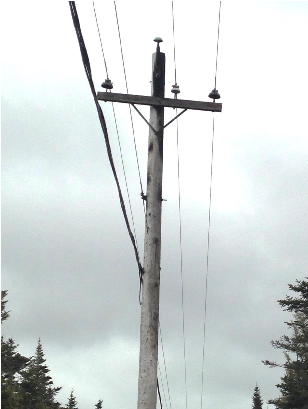
Figure 5 – Damaged Pole Due to Failed Insulator
