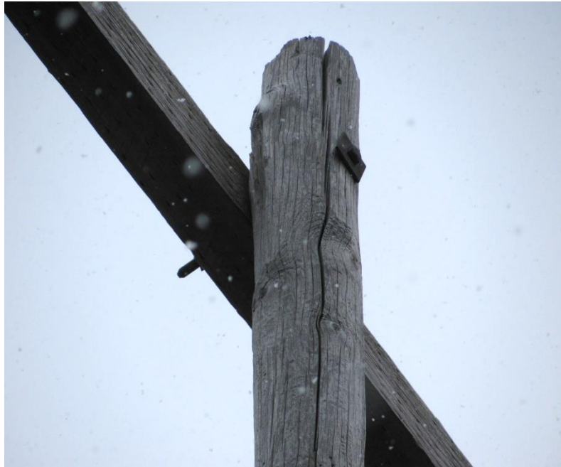
Figure 12 – Severe Check in Pole Top
