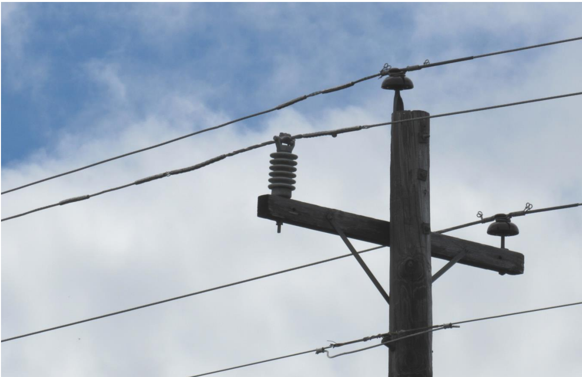
Figure 5 – Damaged Conductor/Pole and Crossarm Deterioration
