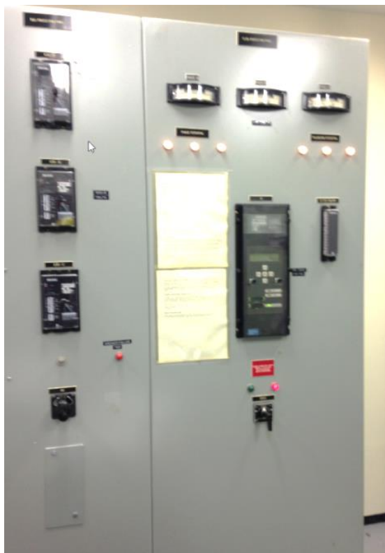
Figure 6: Existing Control Building with Electromechanical Relays
