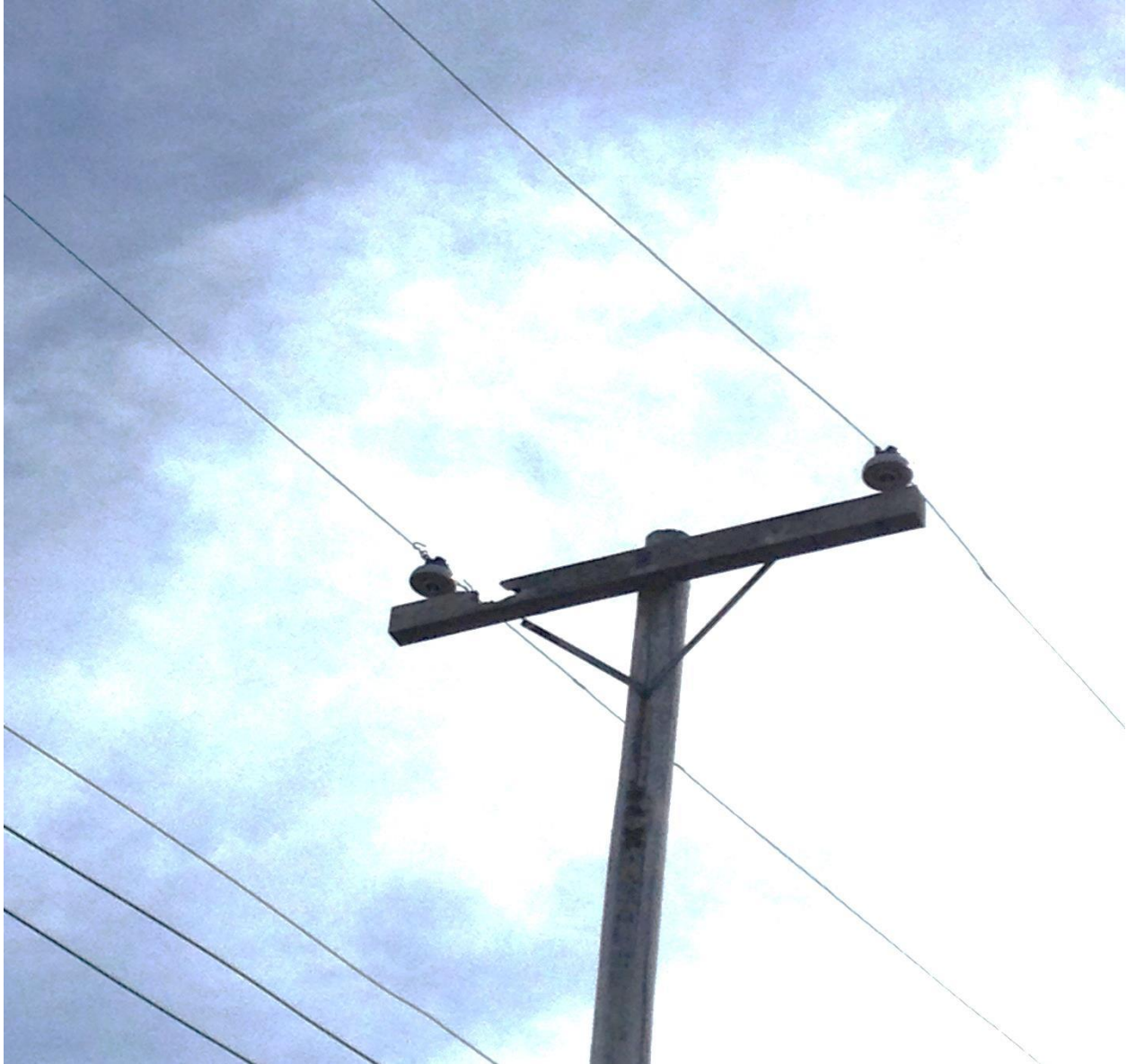
Figure 6 – Damaged Crossarm Due to Failed Insulator
