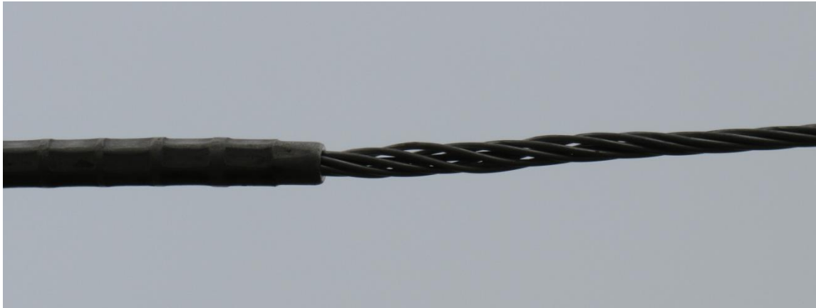
Figure 8 – #2/0 ACSR Conductor Bird Caging
