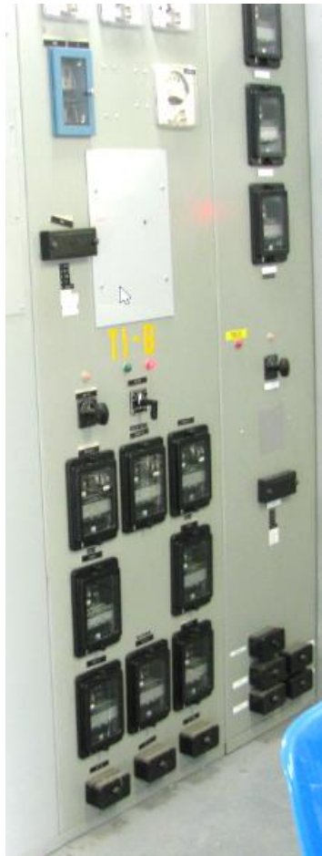
Figure 12: Existing CHA Control Building with Electromechanical Relays
