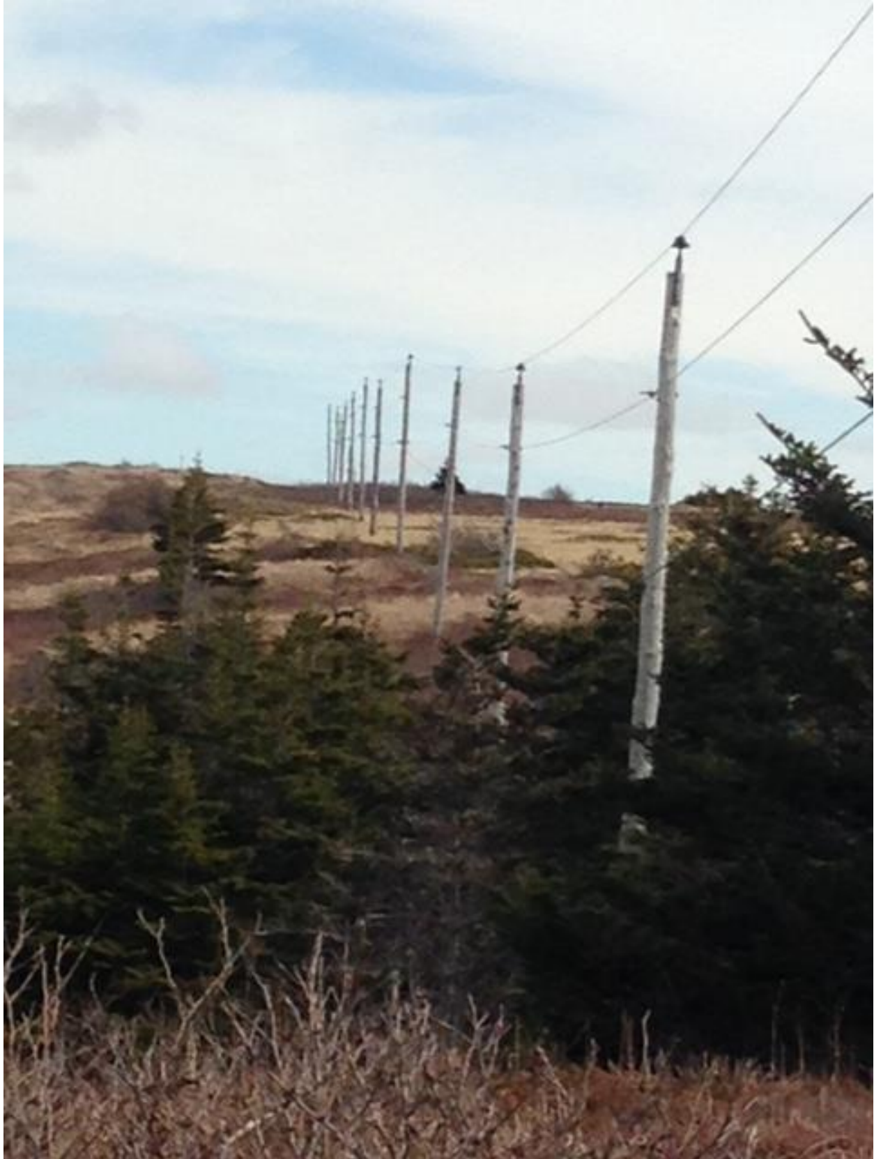
Figure 3 – Non-Standard 1960's Vintage Construction on 30' Poles
