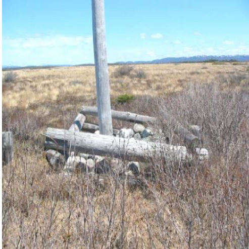
Figure 3: Pole Crib Requiring Repairs
