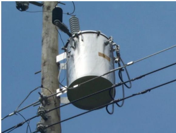
Figure 13: Stainless Steel Pole Mounted Transformer
