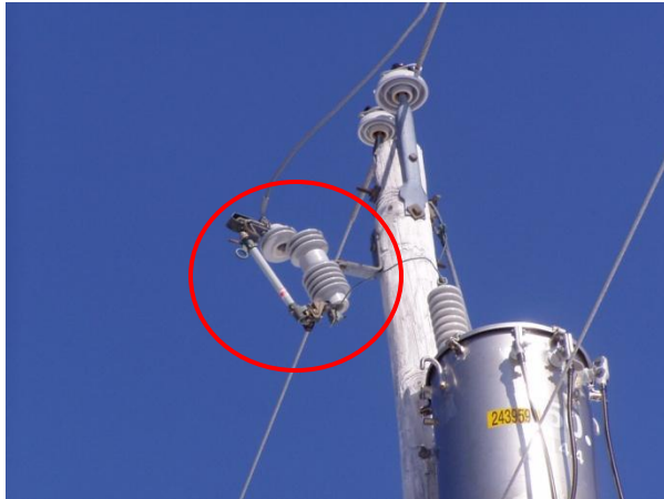
Figure 11: Broken Porcelain Cutout In Service
