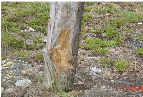
Figure 1: Damaged Wooden Pole
