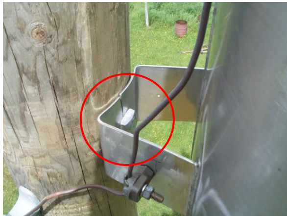
Figure 14: Broken Stainless Steel Transformer Hanging Bracket
