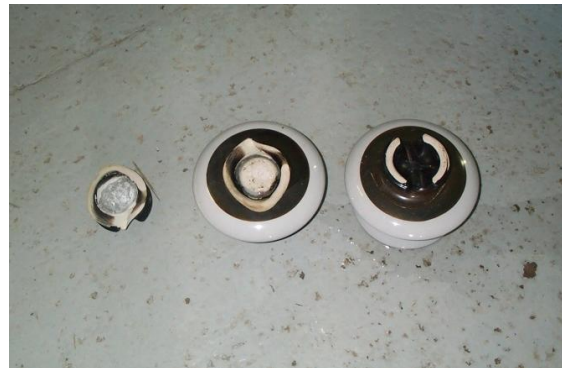
Figure 7: Broken Insulator Removed From Service
