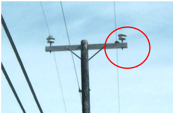
Figure 6: Broken Insulator In Service
