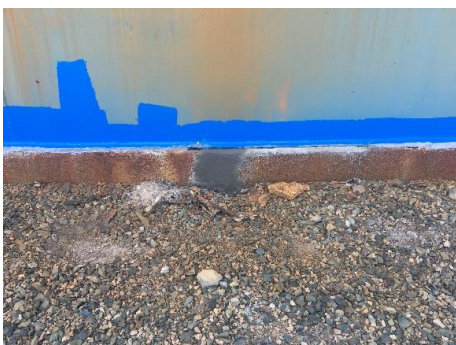
Figure 5: View of concrete repair and sealant applied to tank chine and ring beam interface.
