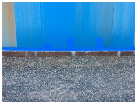
Figure 6: View of concrete repair and sealant applied to tank chine and ring beam interface.
