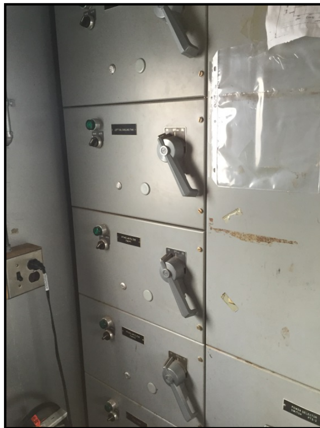
Picture 12: Motor Control Center
