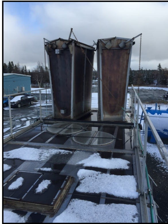
Picture 5: Exhaust Stacks
