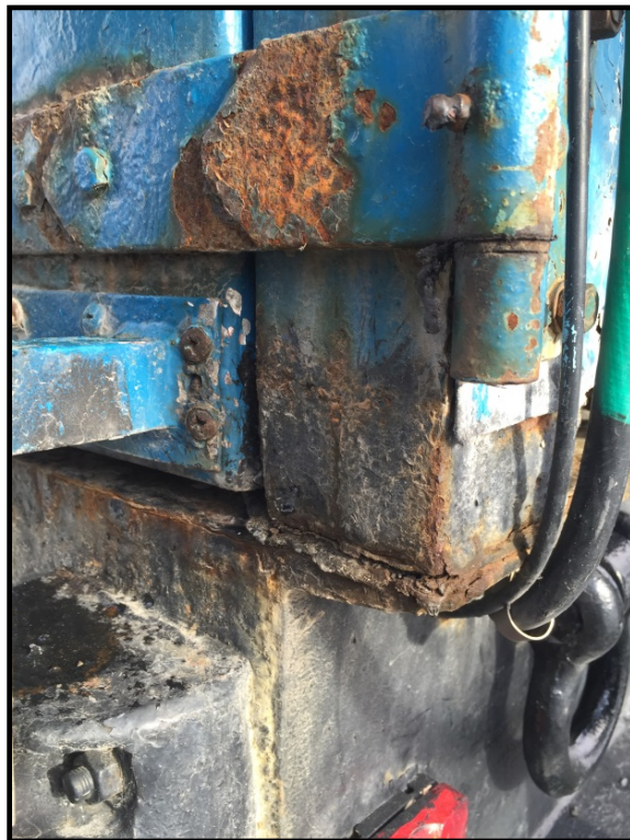
Picture 14: Enclosure Condition
