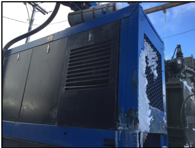
Picture 6: APU Enclosure
