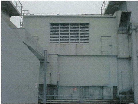
Top Air Box & Bus Duct
