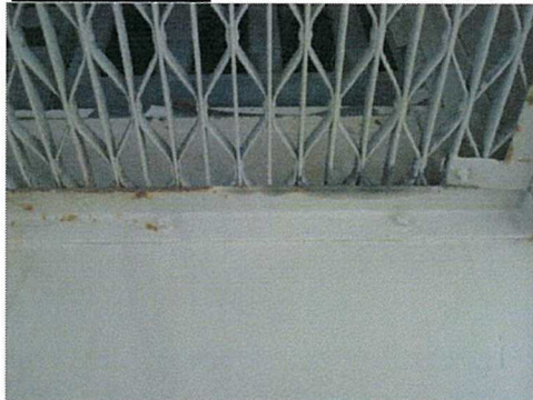
Air Box Walkway
