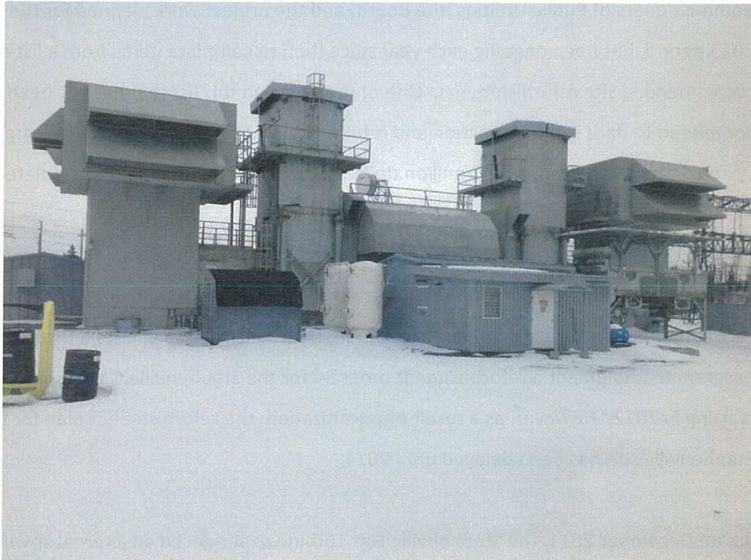
Figure 1: Hardwoods Gas Turbine Plant
