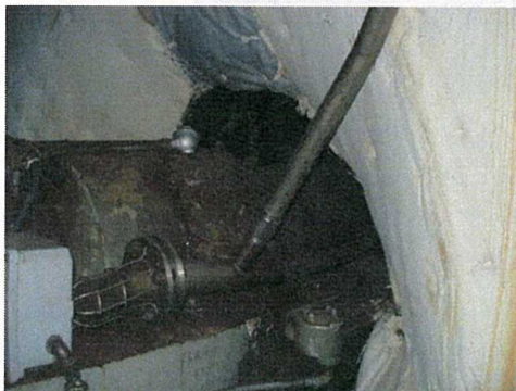
Exciter End Exhaust Insulation
