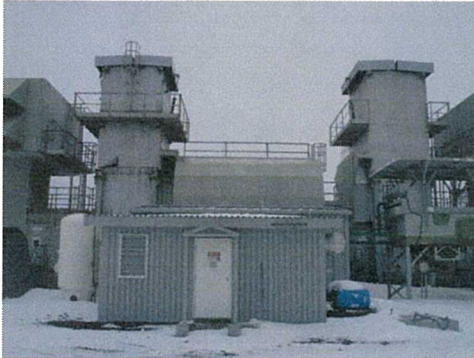
Lube Oil Pump House
