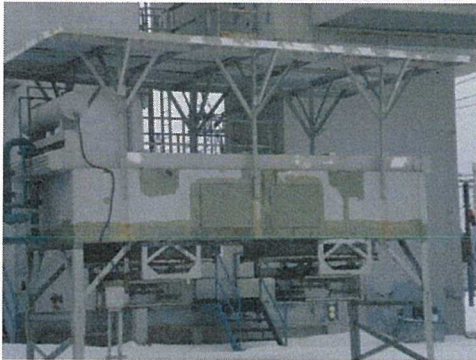
Lube Oil Cooler
