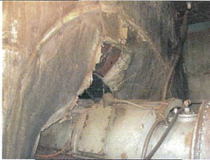
Drive End Exhaust Insulation
