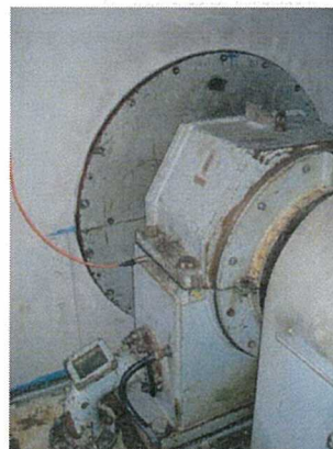
Exciter End Bearing Pedestal
