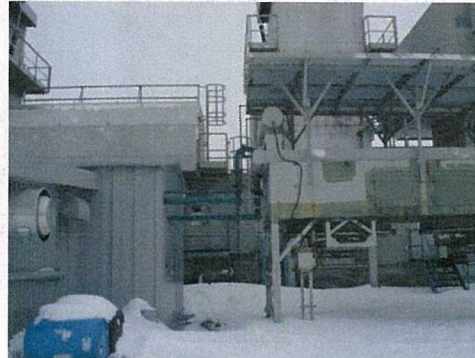
Lube Oil Cooler Pipes
