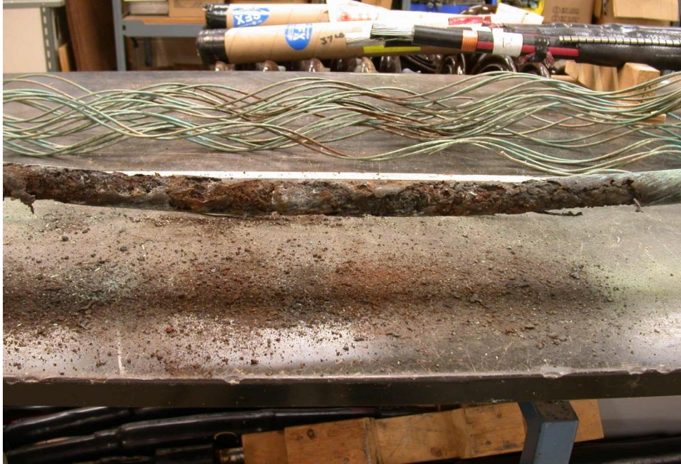
Figure 12: Failed cable after the removal of armor wires showing corrosion powder.
