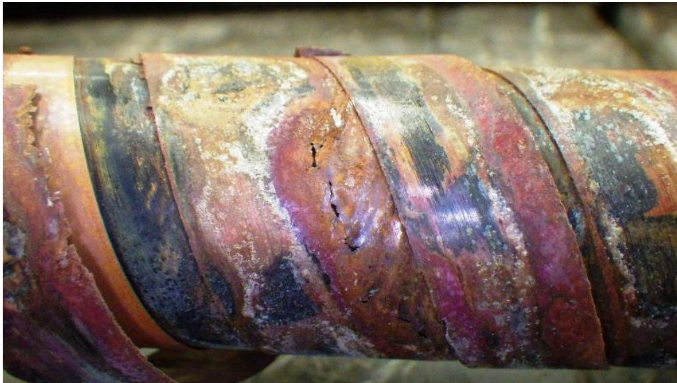
Figure 15: Perforations on the copper tape of Sample #1 of the failed cable.
