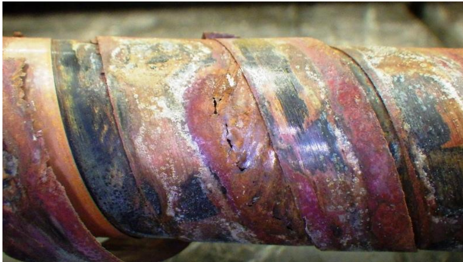
Photograph 4 – Perforations and corrosion of copper tape on faulted cable.
