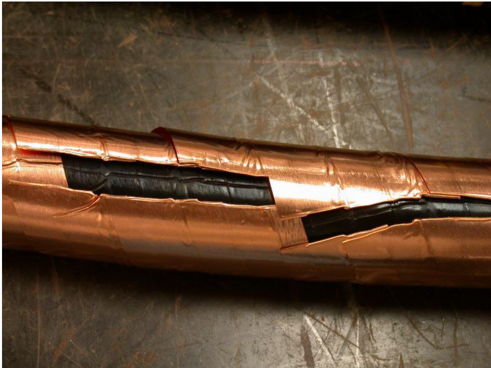
Figure 5: Cracks in the copper tape of spare cable Reel # ADG 1065.
