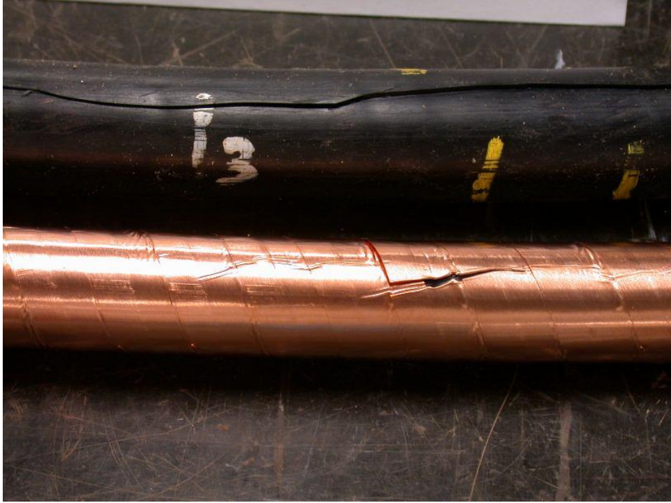
Figure 4: Cracks in the copper tape of spare cable Reel # ADG 1065.
