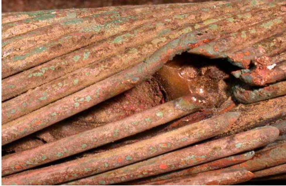
Figure 10: Closer view of the faulted location.
