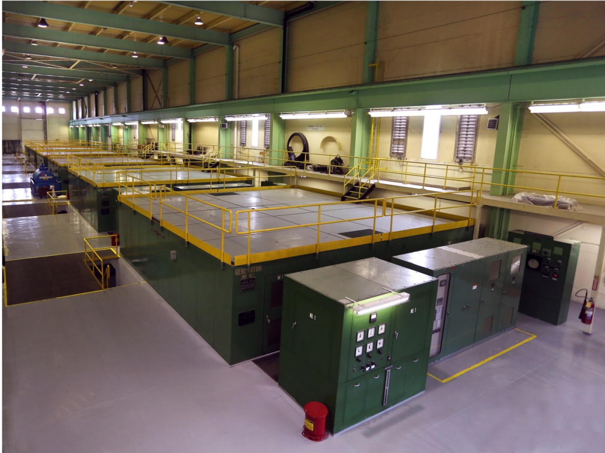
Figure 3: Bay d'Espoir Hydraulic Generating Units 1 - 6
