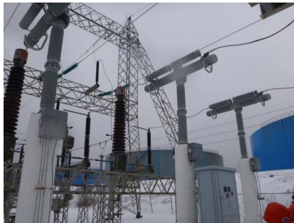
Illustration 3.4: Air-Blast Circuit Breaker B1L17
