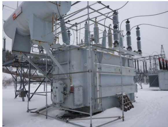
Illustration 3.3: Western Avalon Transformer T5
