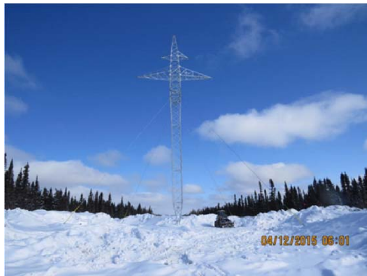
Figure 2, Photograph of a guyed suspension structure used in LIL, conductors were not yet strung 23
