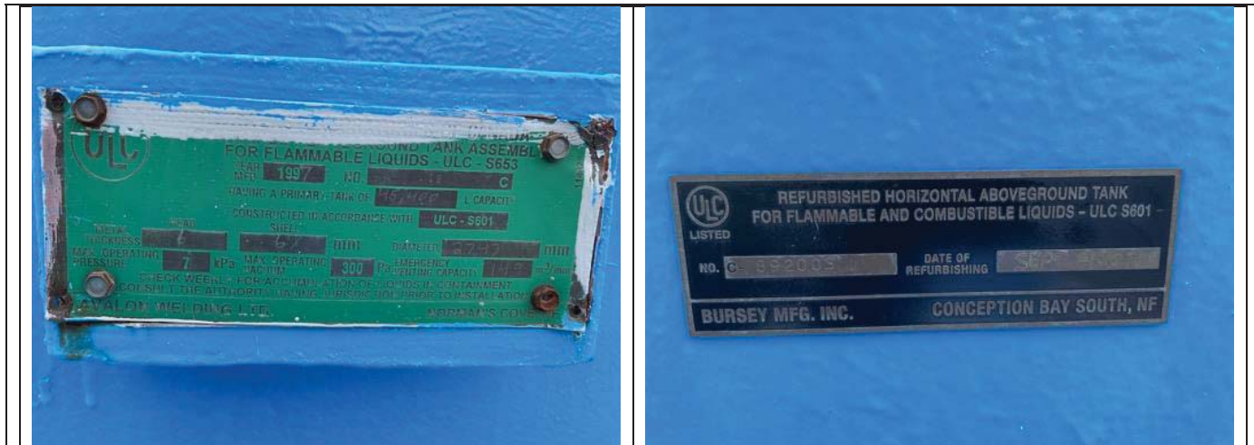
Nameplate partially painted over, refurbish plate above
