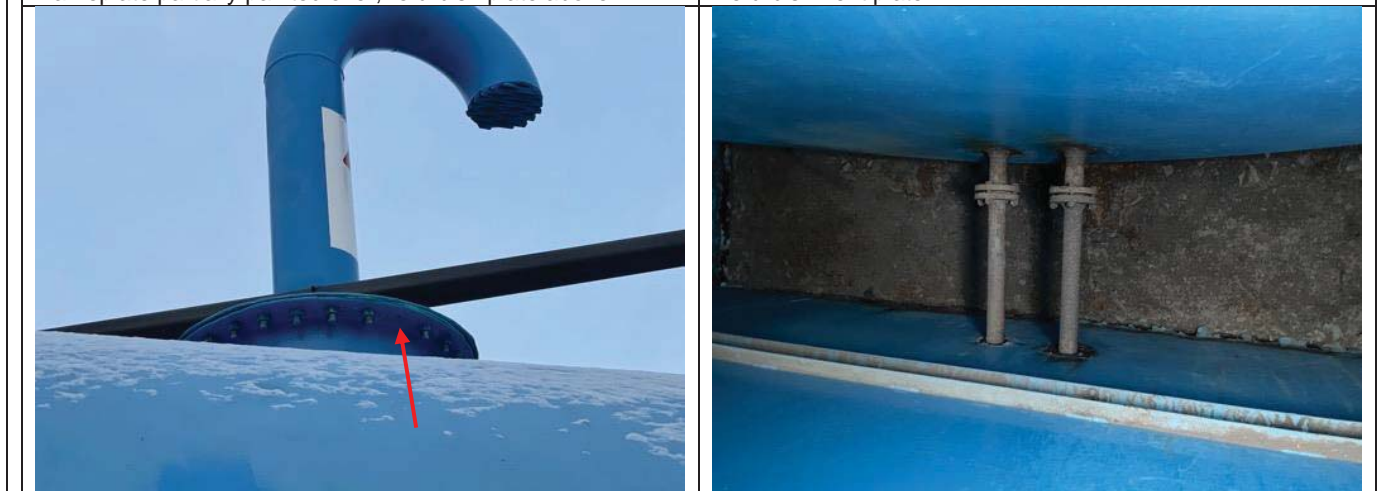
Bolt missing from manway/cover flanged connection
