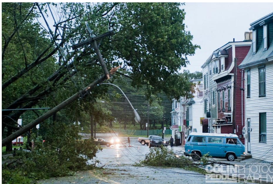
Figure 8: Wind damage to Newfoundland Power distribution line during Hurricane Igor, 2010
