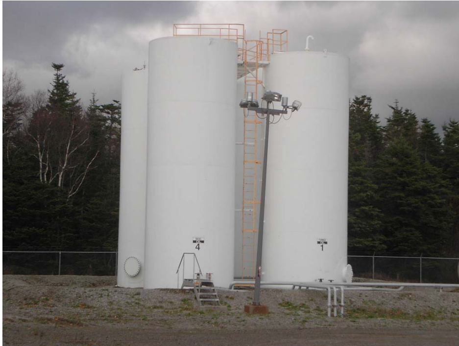
Ultramar – Bulk Plant – Stephenville - Tankage
