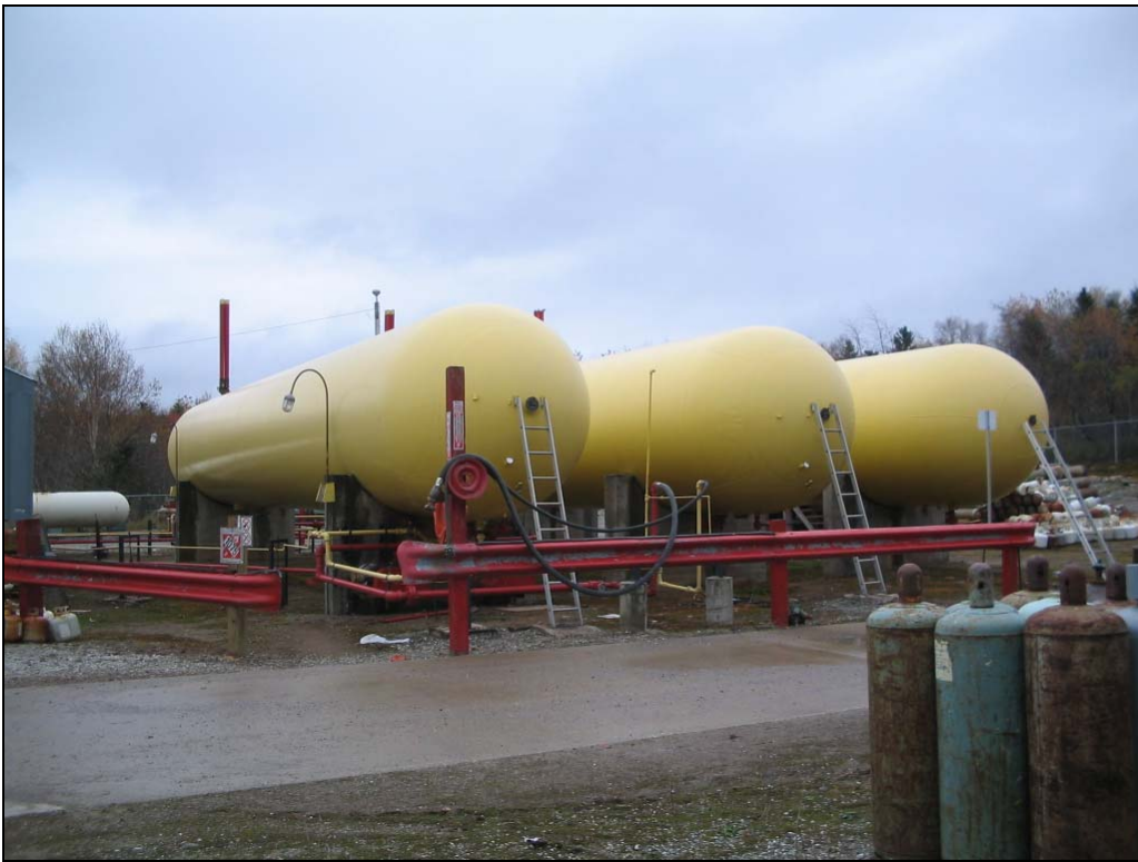
Superior - Propane Storage Plant – Pasadena
