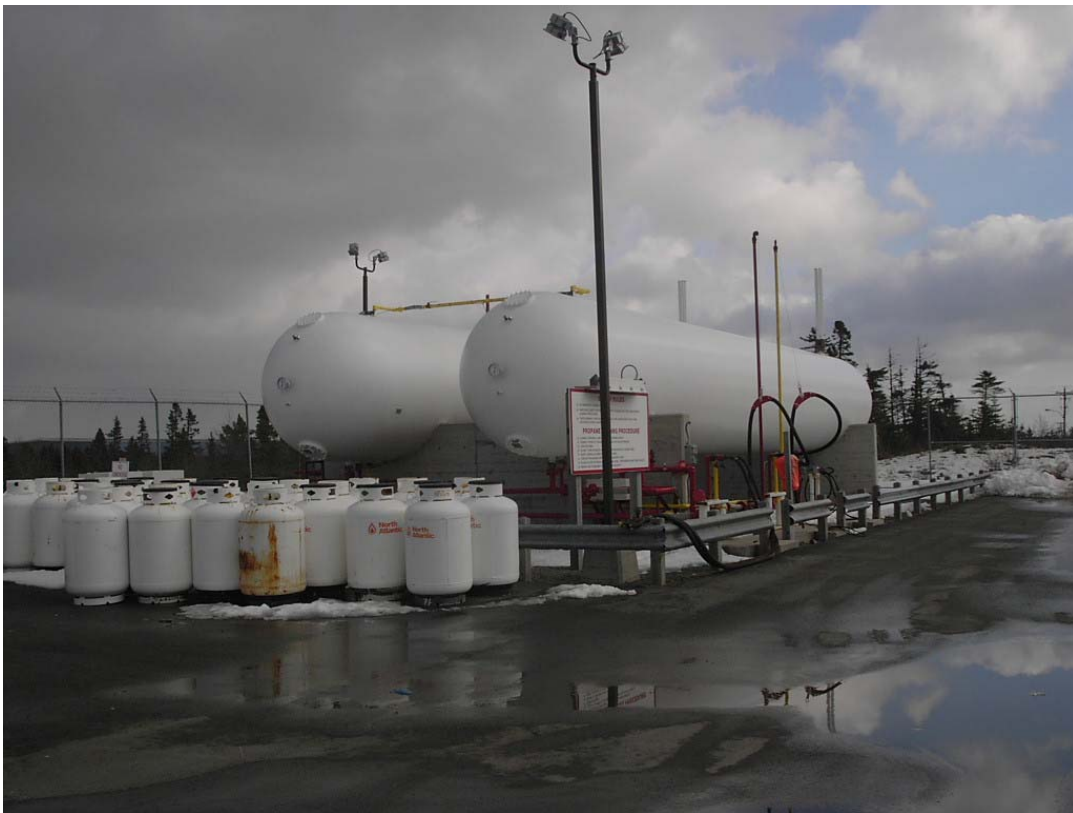
North Atlantic – Propane Storage Plant - Donovans
