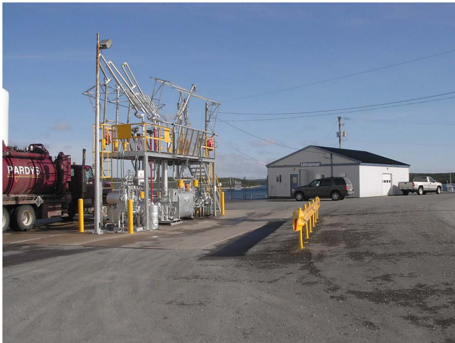
Ultramar – Secondary Marine Terminal – St. Barbe – Loading Rack
