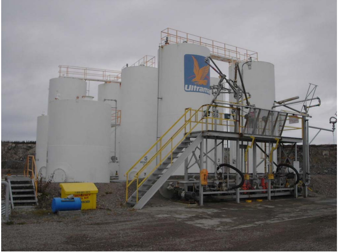
Ultramar Bulk Plant – Fogo Island – Distillate and Gasoline Storage
