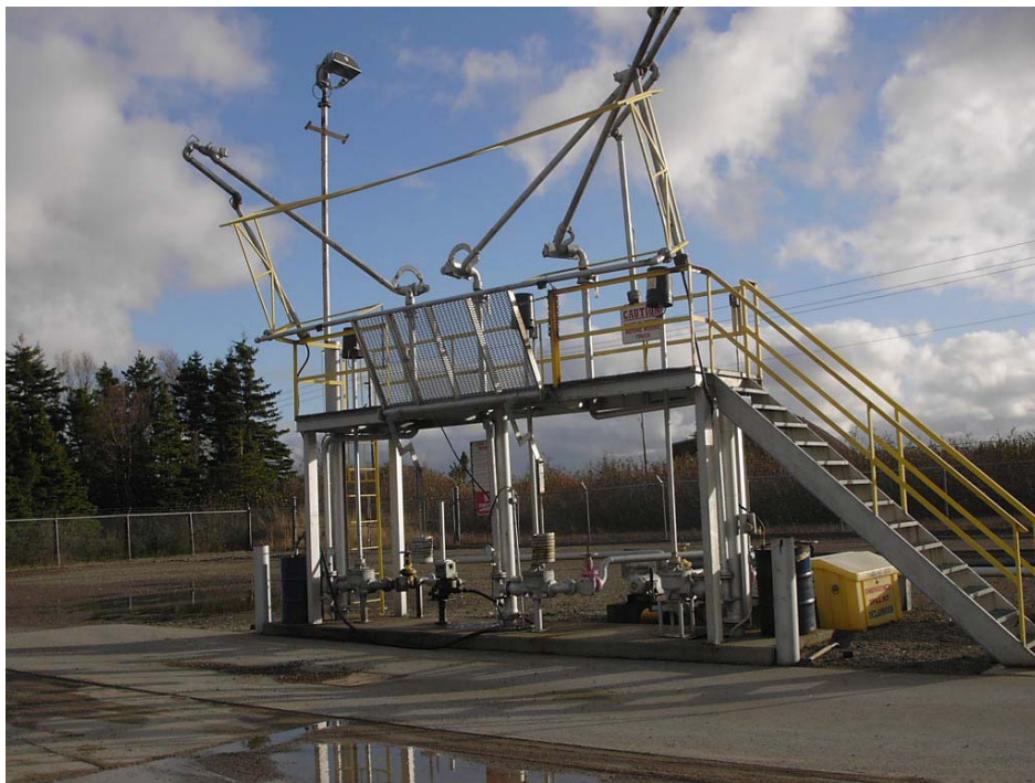
Ultramar – Bulk Plant – Stephenville – Loading Rack
