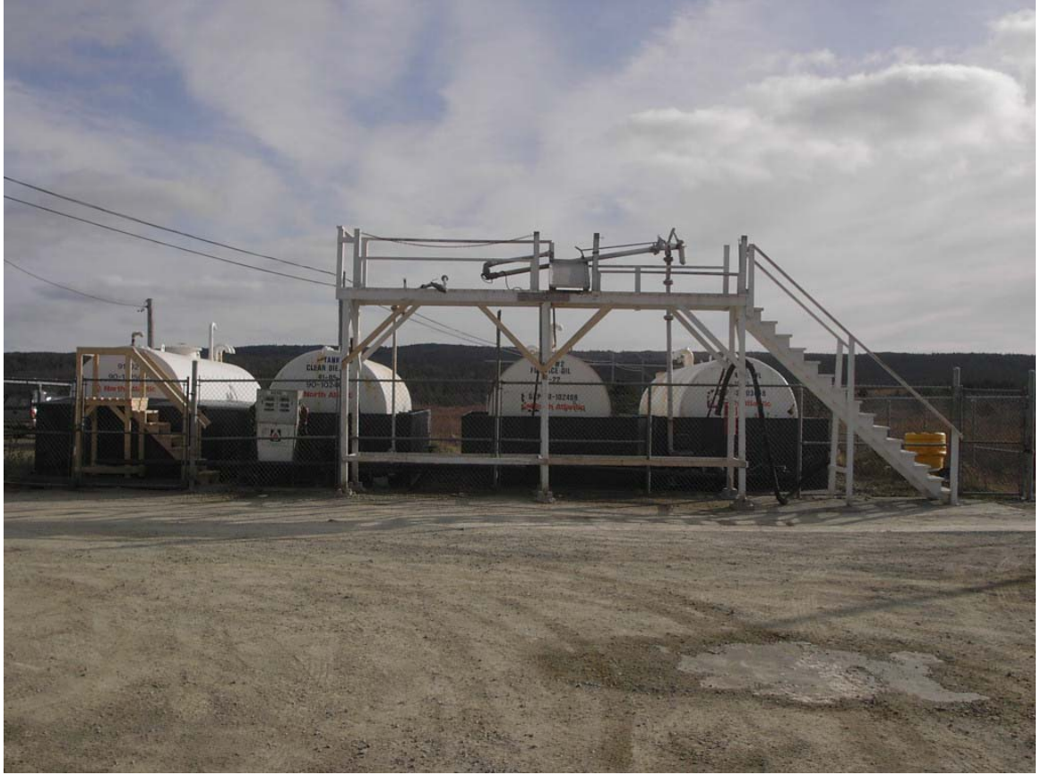
North Atlantic Petroleum – Bulk Plant – Bonavista
