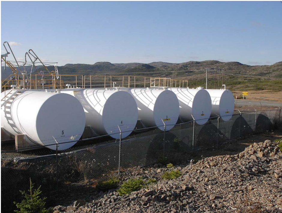
Ultramar-Bulk Plant-Connaiyre Peninsula-Gasoline and Distillate Storage
