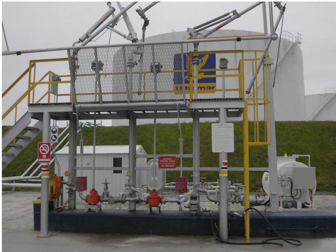
Ultramar Bulk Plant – Loading Rack – Harbour Grace
