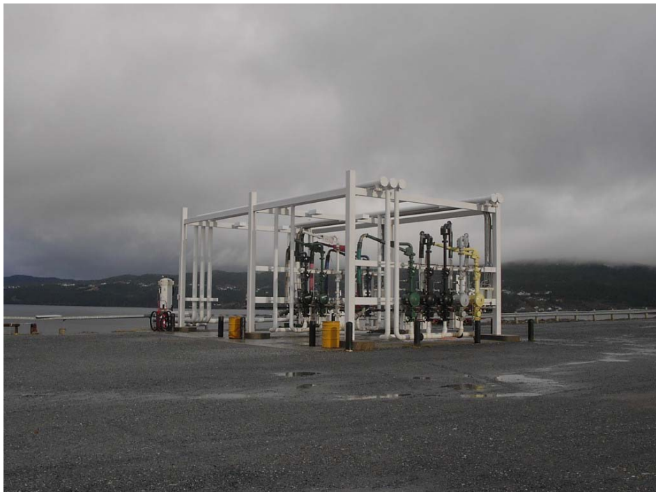
Irving Oil – Marine Terminal – Corner Brook – Loading Rack
