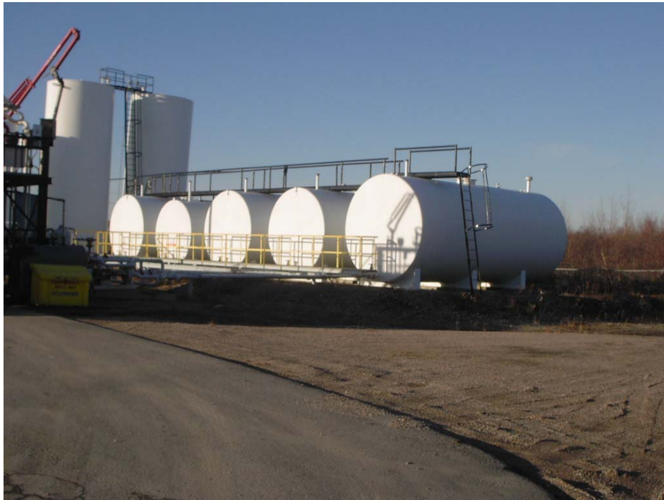
Ultramar – Bulk Plant – Gander (Distillates and Gasoline Storage)
