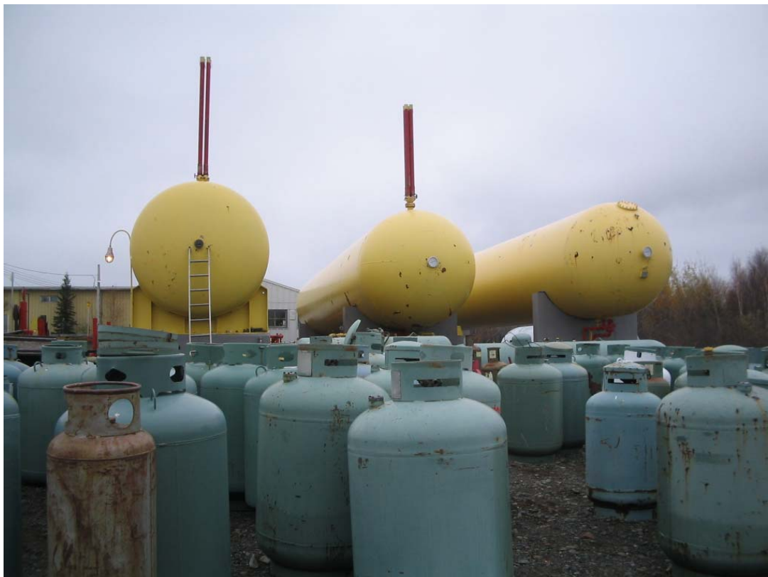
Superior – Propane Storage Plant – Grand Falls-Windsor
