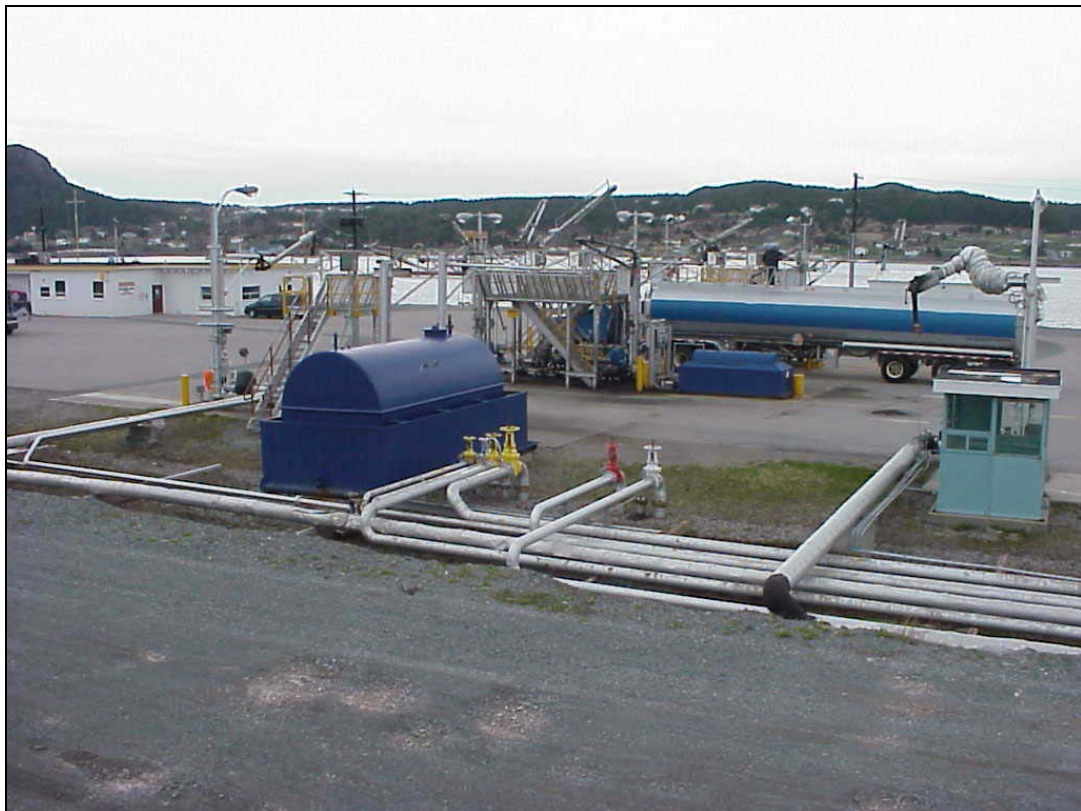
Ultramar Holyrood Terminal – Loading Rack
