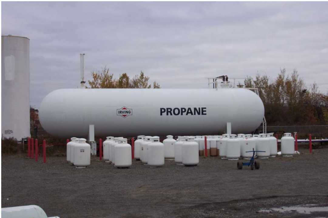
Irving – Propane Storage Plant – Grand Falls-Windsor
