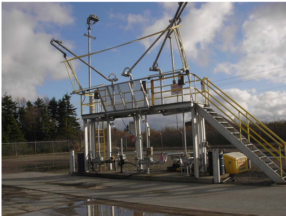
Ultramar – Bulk Plant – Stephenville – Loading Rack
