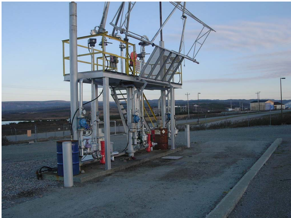
Ultramar – Bulk Plant – Port aux Basques – Loading Rack
