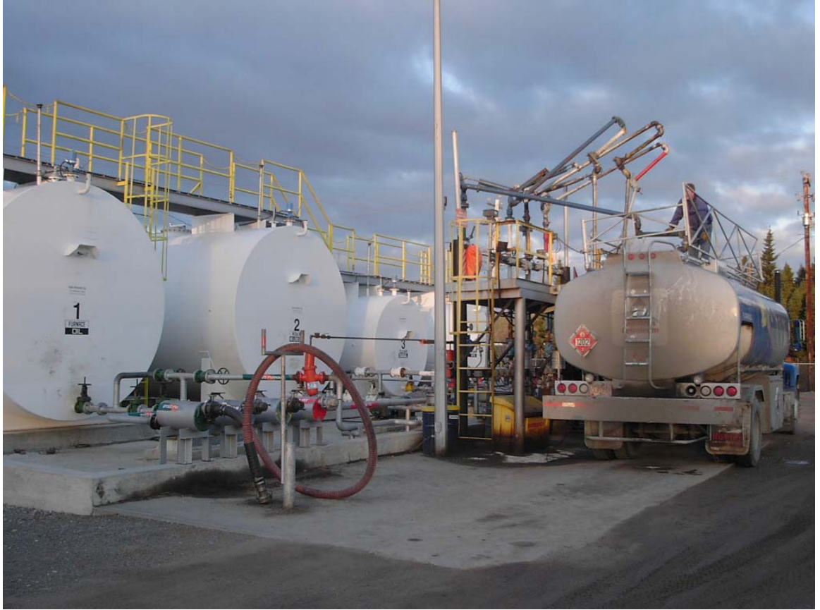
Ultramar – Bulk Plant – Springdale – Gasoline and Distillate Storage
